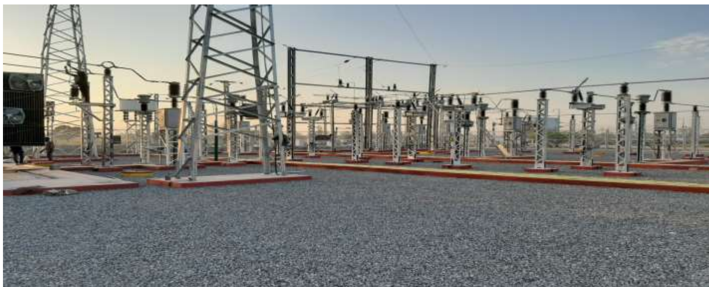
CONTROL WIRING OF OUTYARD EQUIPMENTS ( LV CB, CAPACITOR BANK CB, BM ,BX)
